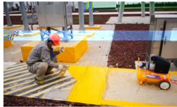
On July 12, 2018, the maintenance personnel of Xinghe Wind Farm of Longyuan Inner Mongolia Company carried out the warning and marking paint for yellow and black in accordance with the requirements of safety and civilized standardization.
