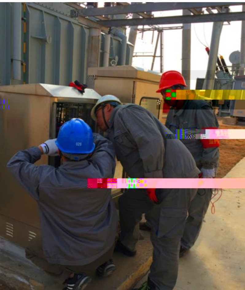
Longyuan Neimenggu Company enhance their equipment defect treatment as shown in the picture of Saiwusu wind farm booster station.
