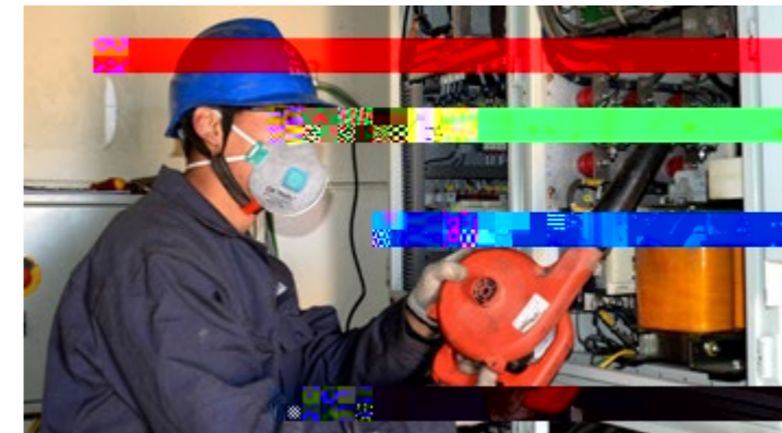
In order to further strengthen the operation status management of wind turbines, timely identify and eliminate hidden defects and ensure the safe and stable operation of wind turbines, the Longwan Hebei Company Dongwan Wind Farm inspectors cleaned and maintained the fan inverters on March 22, 2018
